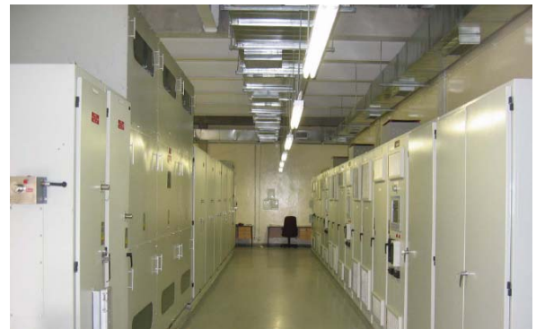
Fig. 2 Adjustable speed drive (left), excitation and control panels (right)
